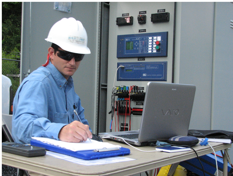
Figure 33. Commissioning of protective relays on site (photo courtesy of Elect PC).
